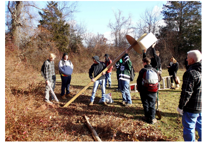
Guilford High School students helped with building and installing Barn Owl nest boxes.
